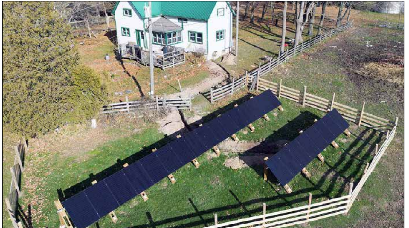
An aerial shot of the Tribe family's 9.720 kilowatt solar panel array.
