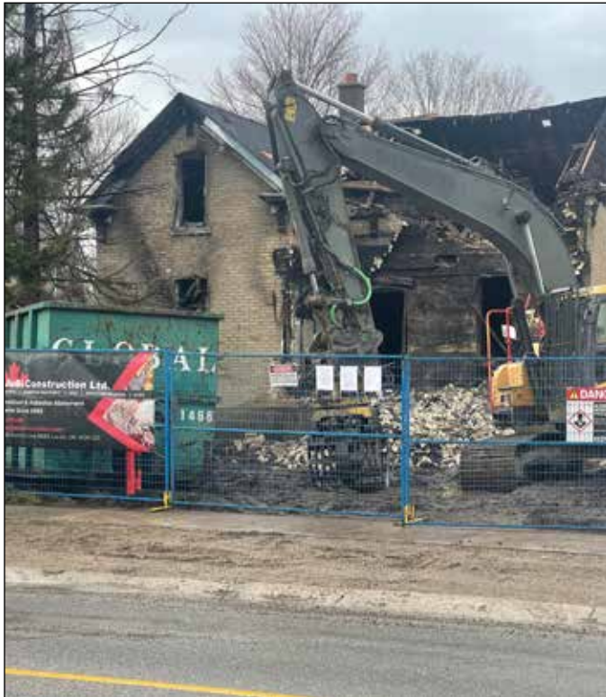
(GARY WEST PHOTO) Crews from JoBi Construction Ltd. of Lucan use heavy equipment to demolish the remains of a two-storey brick home on Woodstock Street North in Tavistock last week. Neighbours welcomed the cleanup, saying the fire-damaged structure had become both an eyesore and a potential safety concern.
