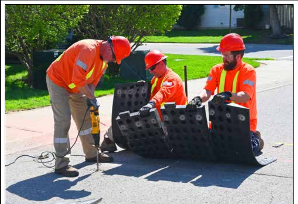
BUMPETY BUMP Workers with the town's roads department were busy on Monday installing speed bumps on Wilson Ave as a traffic calming measures. Following complaints from residents about speed and that the existing radar speed signs weren't working, council approved the speed bumps. These will be removed in the winter so as not to hinder snow plowing.
