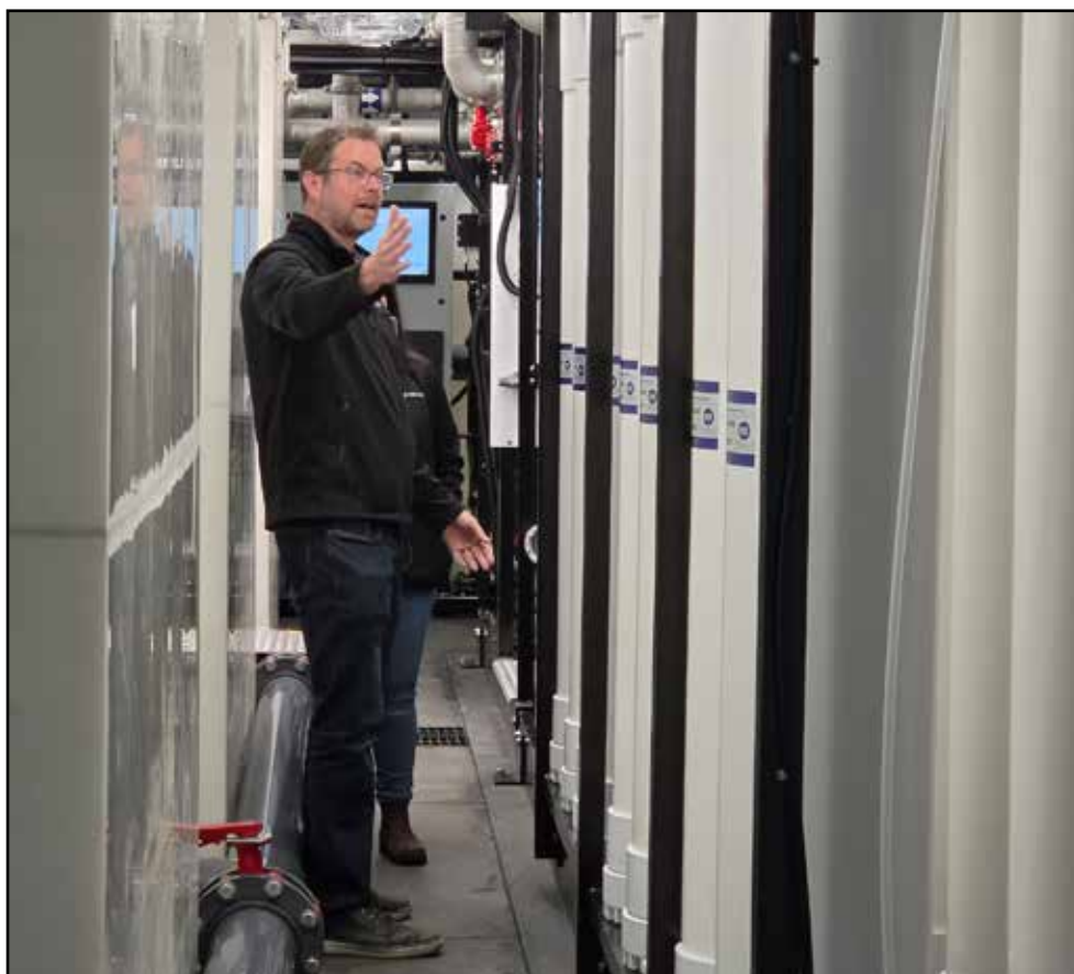
Fraser Kent, CEO of Laminar Water in Cambridge, gave the media a tour of the first of four water-treatment units, which will be installed at the Mannheim water treatment plant to boost water capacity in the region. Each unit comes with a price tag of about $2 million.
